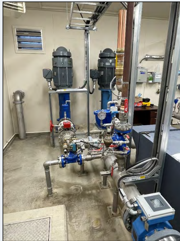
Treatment Station Booster Pumps
